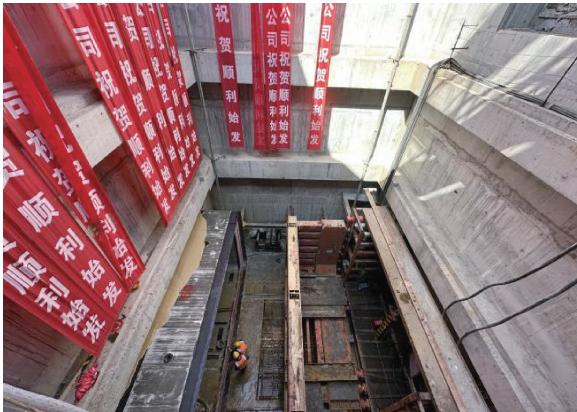
图 1 矩形顶管破洞图 Fig. 1 Picture of rectangular pipe jacking hole
